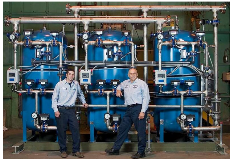
Triple 48" Diameter Softener System with Optional Stainless Steel Butterfly Valves, Piping, and Instrumentation
