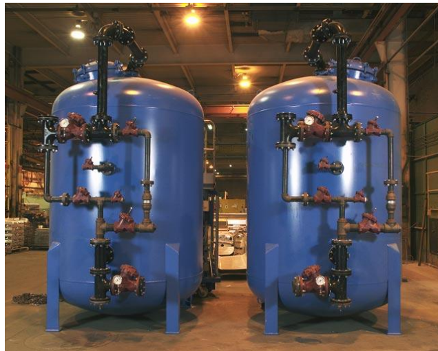
Dual 84" Sand Filters with Standard Diaphragm Valves and Steel Piping
